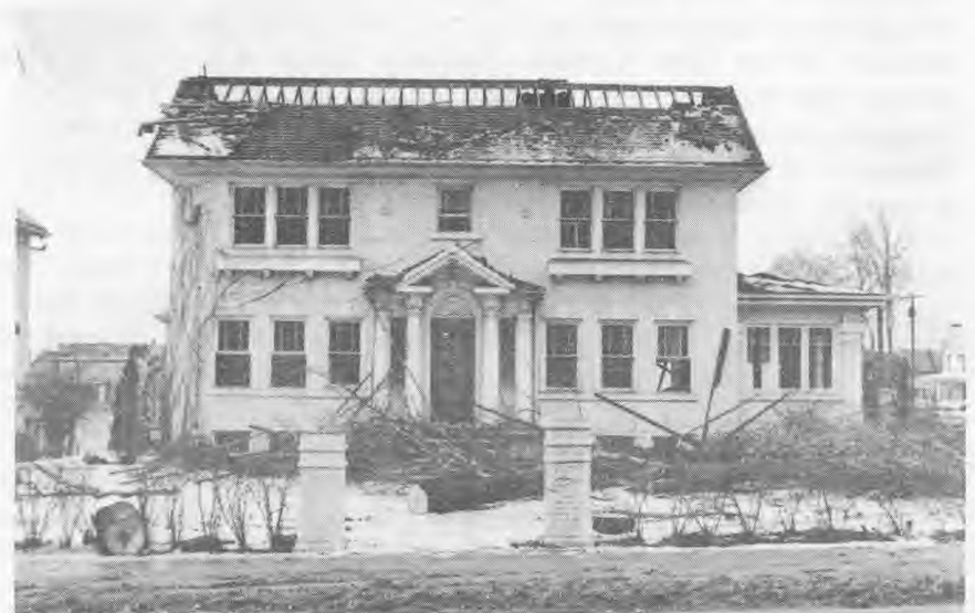
Home of Burt M. Allen, former mayor of Rockford, in the process of being torn down. See page 7 for complete story.
